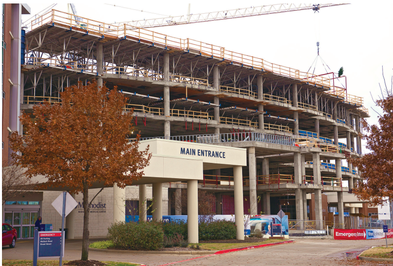
A crane lifts the final beam — topped with an evergreen tree — into place as construction crew members prepare to secure it to the highest structure of the new patient care tower.
